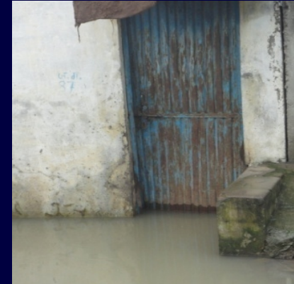
Water enters low-plinth house after heavy rain: climate change
